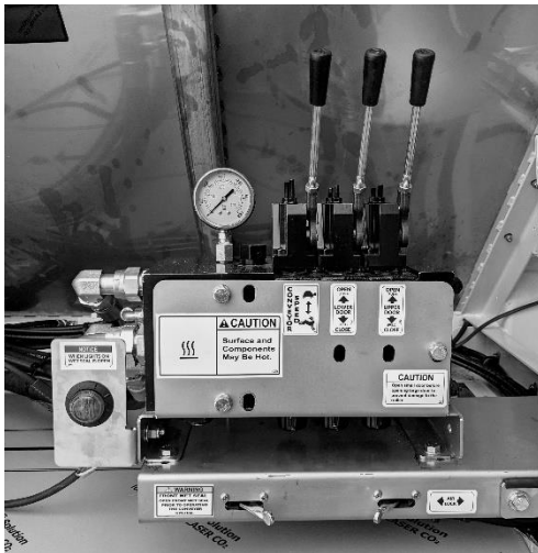
Figure 122- Manifold with wet seal and air lock flipper valves. .
