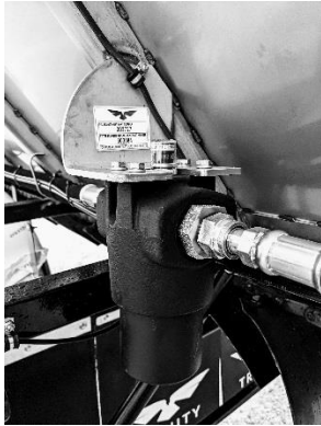
Figure 48- High Pressure Filter Location
